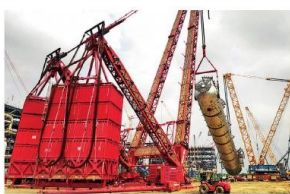
• Erection of 1370 MT equipment by 3200 MT crane and 1600 MT trailing crane at Bathinda Refinery of HPCL-Mittal Energy Ltd (2020)
