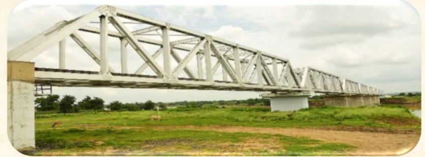
Fabrication and Launching of open web through girders for major bridges between Jhalawar-Aklara section for W.C.
