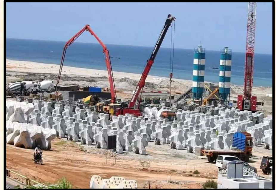
Casting and Staking of Accoropodes for break water development of Vizhinjam Port at Kerala of Vizhinjam International Seaport Ltd. For Adani Group
