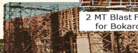
Civil Works for 3 X 200 MW Thermal Power Station at Obra for U.P.S.E.B
