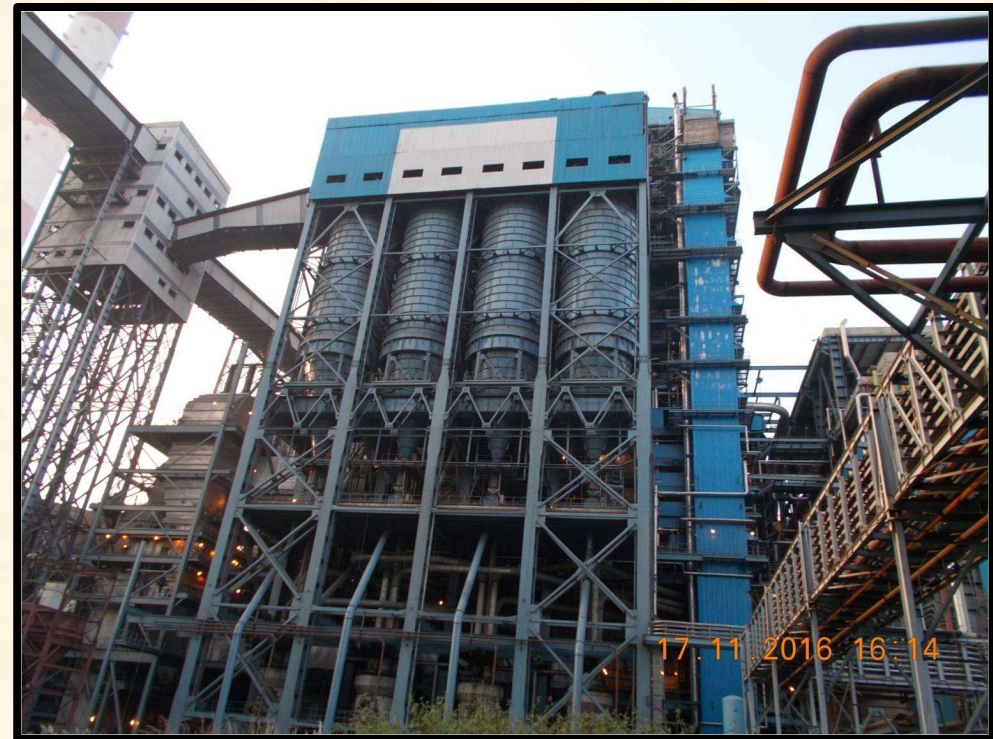
LHS Bunker at 2 X 500 MW Units at Sagardighi STPP of West Bengal Power Development Corpn. Ltd.
