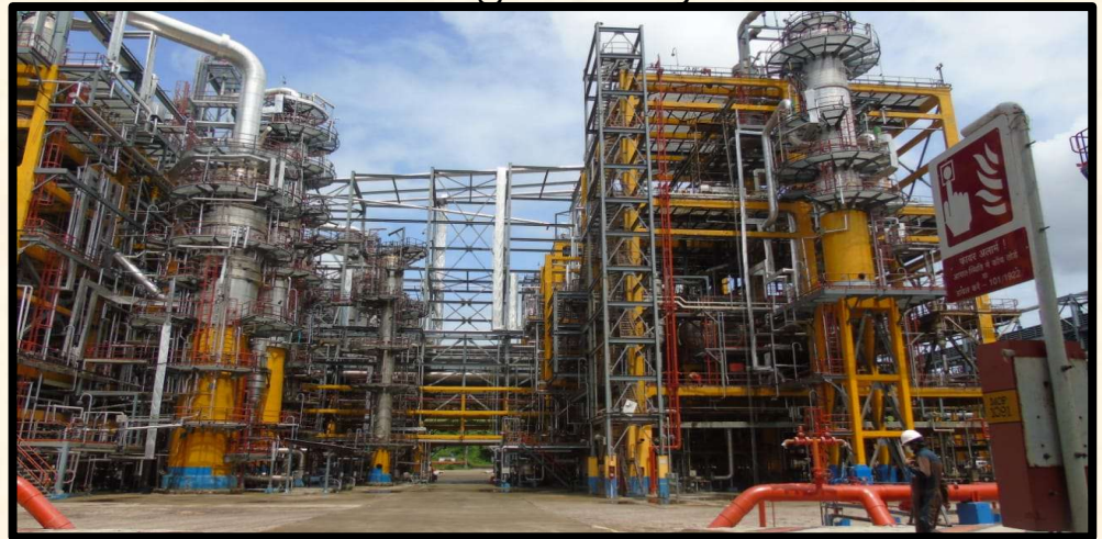
Acrylate Unit at BPCL Kochi Refinery
