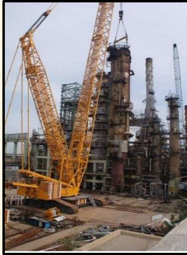
CDU VDU-II Revamp Project at Chennai Petroleum Corpn. Ltd.
