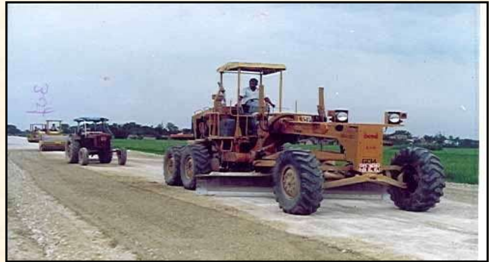
Construction of 2 lanes Durgapur Expressway with grade intersections & repairing of minor bridges & culverts, toll plaza & service road at Dankuni, W.B.) for National Highways Authority of India
