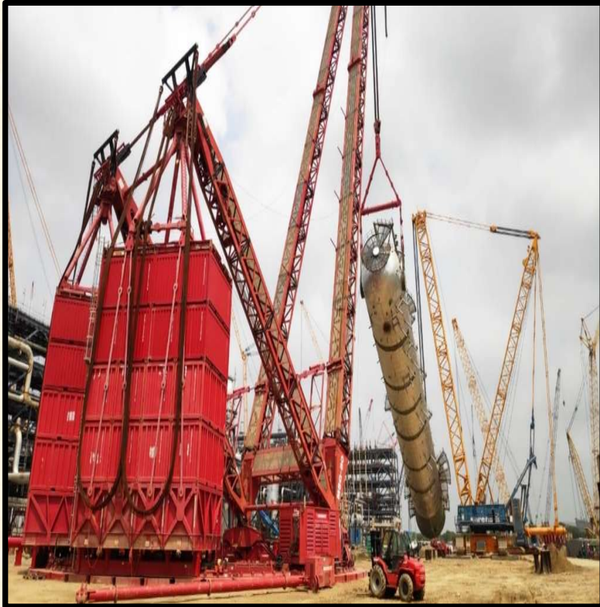
Erection of 1370 MT Equipment by 3200 MT crane and 1600 MT trailing crane at Bathinda Refinery of HPCL-Mittal Energy Ltd.
