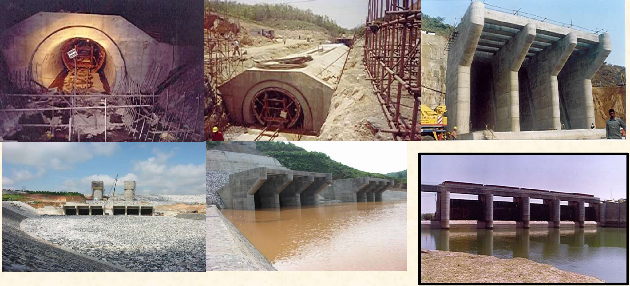
Construction work at Gosunda Dam, Rajasthan of HZL for Tungabhadra Steel Products Ltd.
