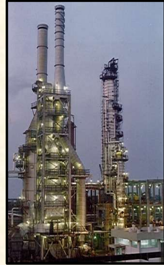
VDU Furnace at IOCL, Haldia
