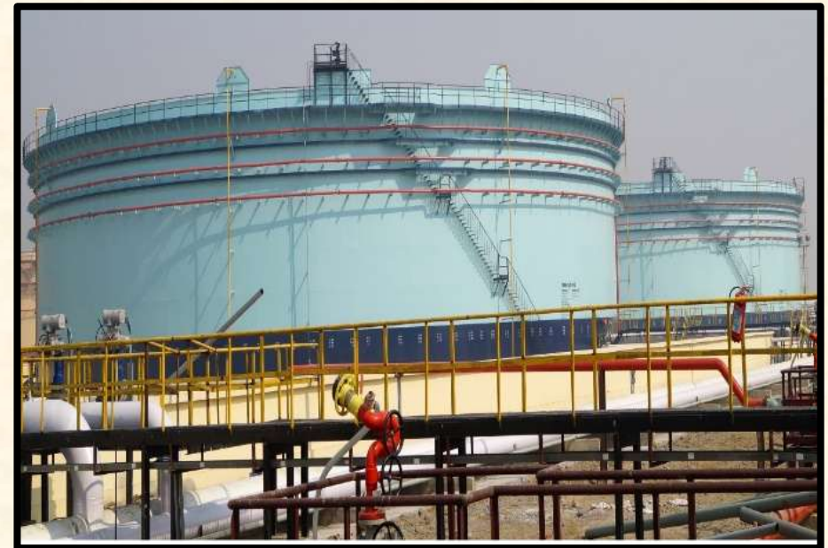
Steel Storage Tanks at Hindustan Petroleum Corpn. Ltd Kanpur Terminal
