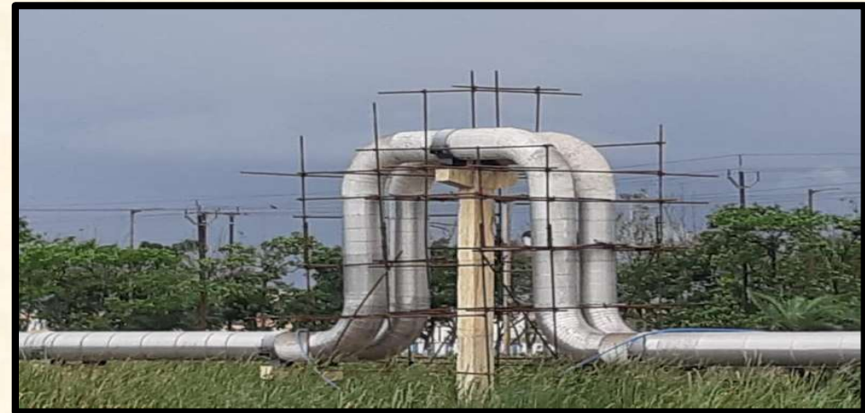
Propane and Butane pipeline Double Wall 18"/25" size Cross-Country Pipeline for BPCL Haldia
