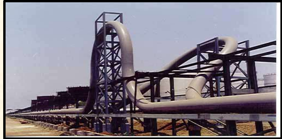
Cross-Country Pipeline for transportation of Black & White Oil for Oil Terminal of Indian Oiltanking Ltd.
