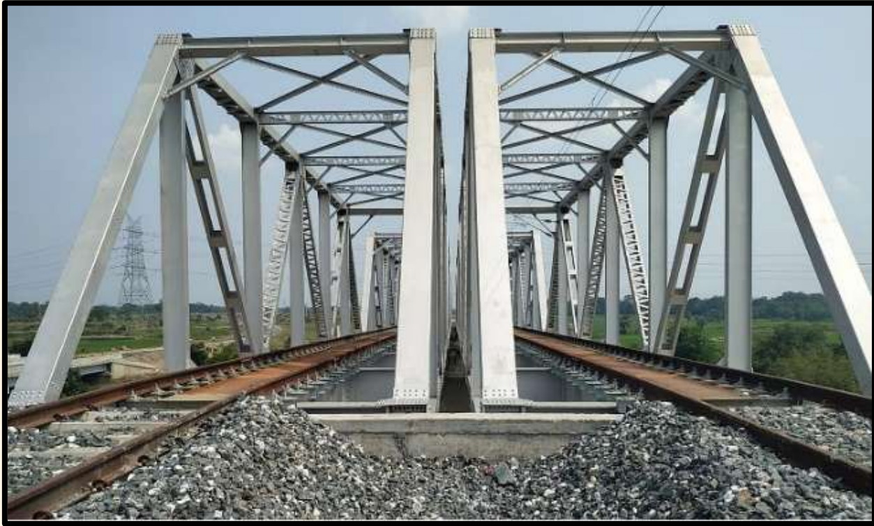
3X2, 30.5 m open web through girder rail bridge over Uthala River at railway siding project of DVC for RITES Ltd. at Raghunathpur
