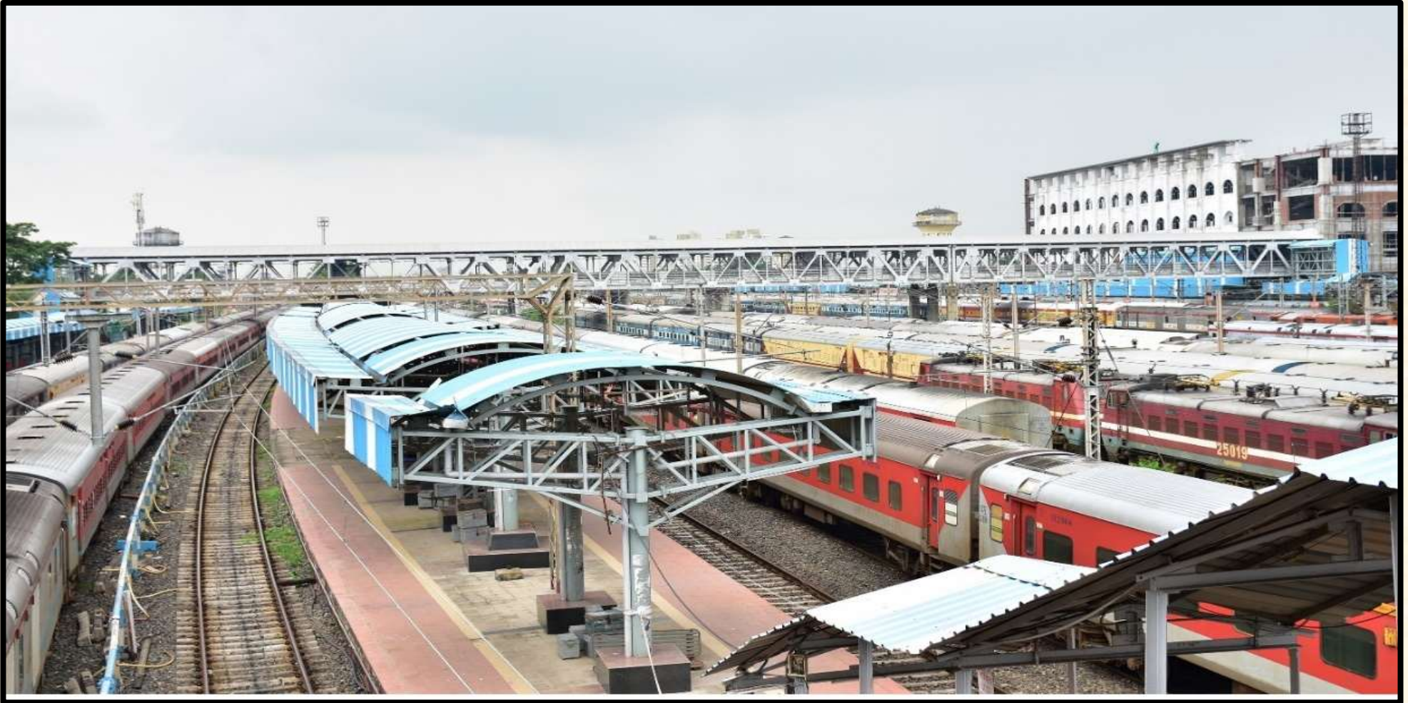
Station Development Work including Foot Over-Bridge of Santragachi Station for South Eastern Railway
