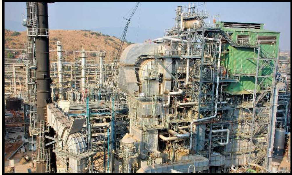
TGTU Unit at Hindustan Petroleum Corpn. Ltd. Vizag Refinery
