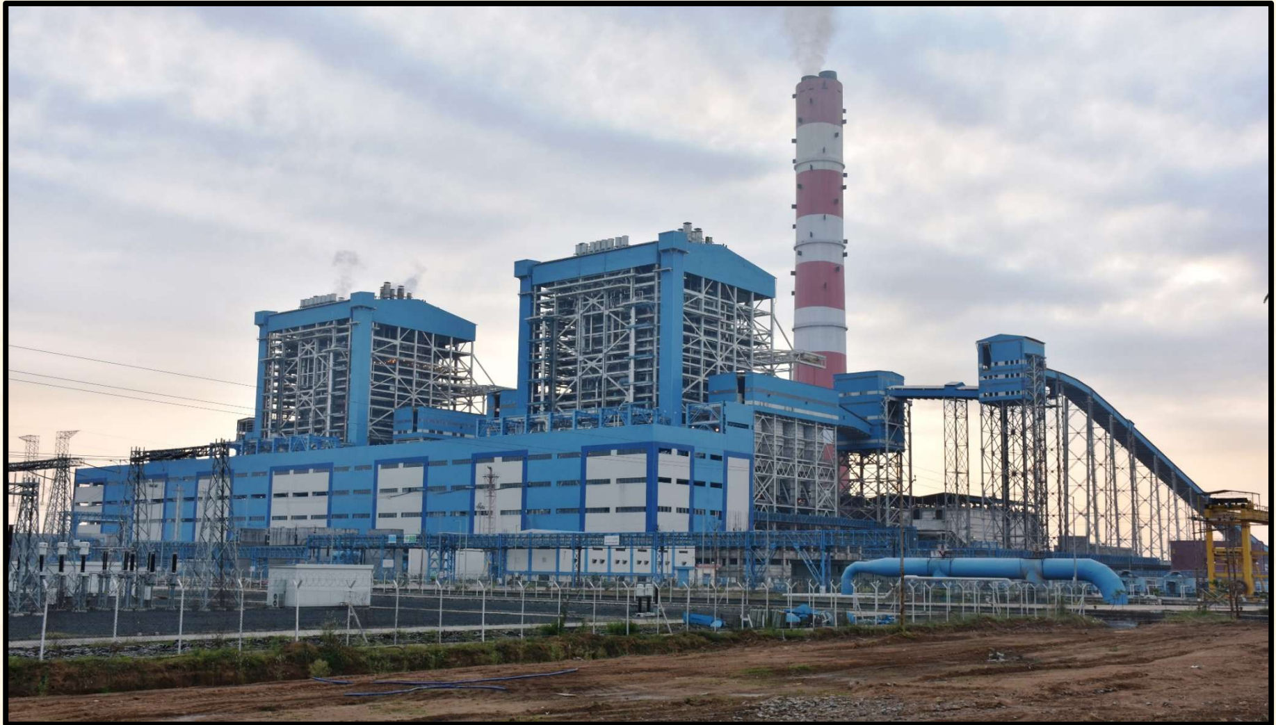
Main Plant and Offsite Civil Works Package for Gadarwara STPP Stage-I (2X800 MW) (including Double Flue Chimney of height 275m & Chimney Elevator) for NTPC
