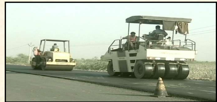
Strengthening and Paving of shoulders : Dholka to Bagodara (Km. 0.000 to Km. 23.000) and Wataman to Pipri (Km. 69.600 to Km. 94.000) for Government of Gujarat
