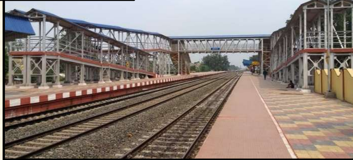
Earthwork in embankment, blanketing, RCC bridges, retaining walls, platforms, other ancillary works including P-Way works in Nimtita-Sujnipara Section for South Eastern Railway
