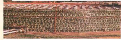
Crude Oil Storage Tank for ONGC, Uran
