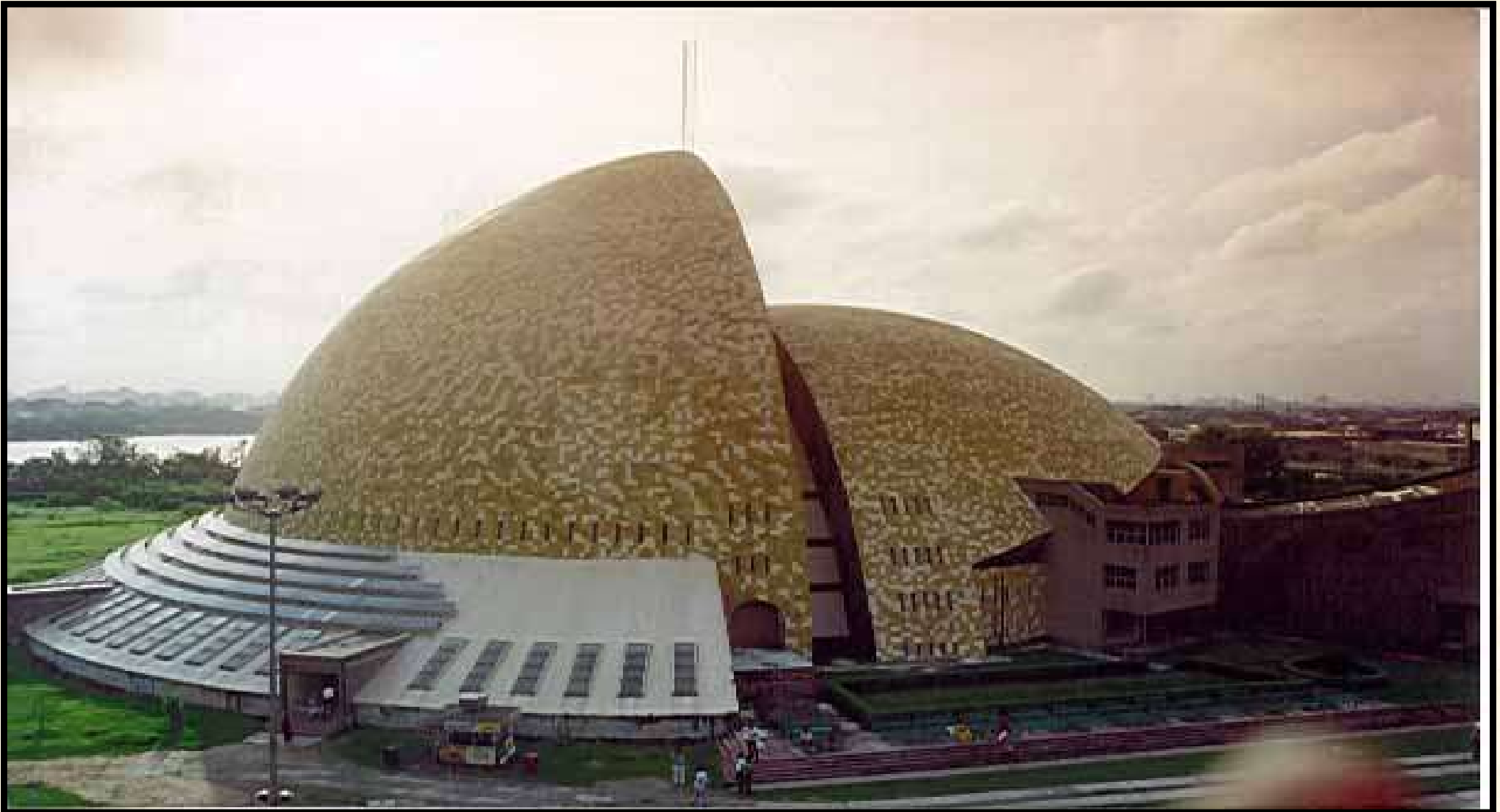
Construction of Convention Centre at Science City, Kolkata for National Council of Science Museums
