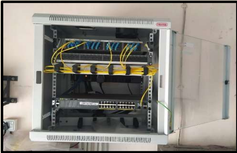
Plant wide Data Network (PWN) and Fire Detection & Alarm (FDA) Monitoring System under Modernization & Expansion of Bhilai Steel Plant (BSP)
