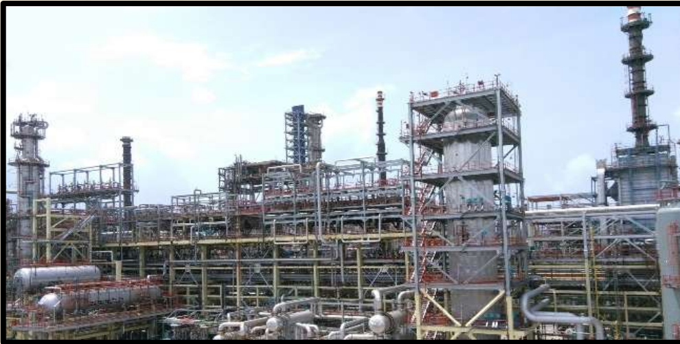
DHT Unit at Bharat Petroleum Corpn. Ltd. Mahul
