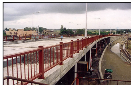
Construction of Flyover over NH-2 at Durgapur for National Highways Authority of India
