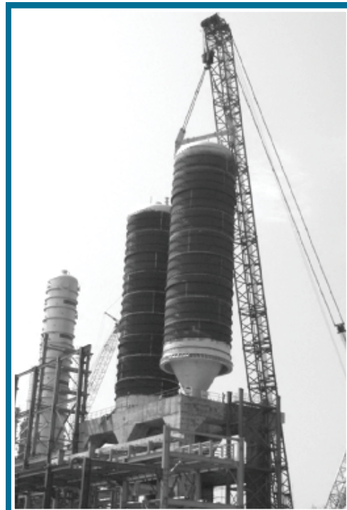
Erection of two nos. Coke Drums of 575 Mt each at CPCL, Chennai
