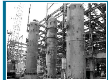
DCU Unit at BPCL, Kochi
