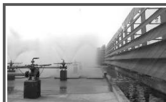
Turnkey execution of Mist Cooling Water System for Gas Cracker Unit at GAIL, Pata
