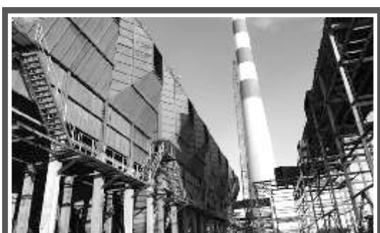
Erection, Testing, Commissioning of ESP, Boiler, and other Auxiliaries at Sagardighi, W.B. for M/s BHEL
