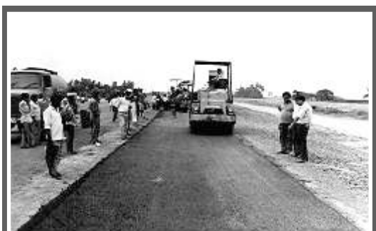
Two Lane Expressway with Service Roads at Dankuni for PWD, West Bengal
